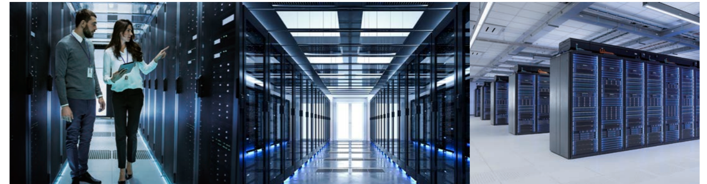
Enterprise/Colocation/Hyperscale Data Center
